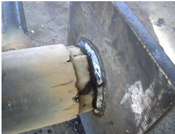
Fig. 7: Full-penetration weld of piles on base-plates, no weld between pile and leg
